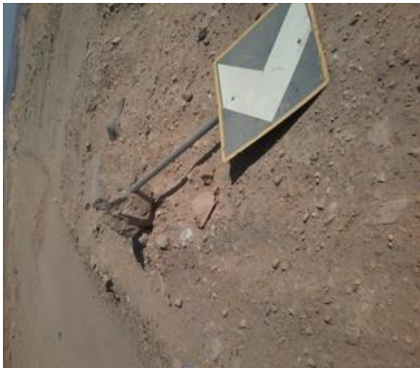
Fig 1. Improper position of road signs.
